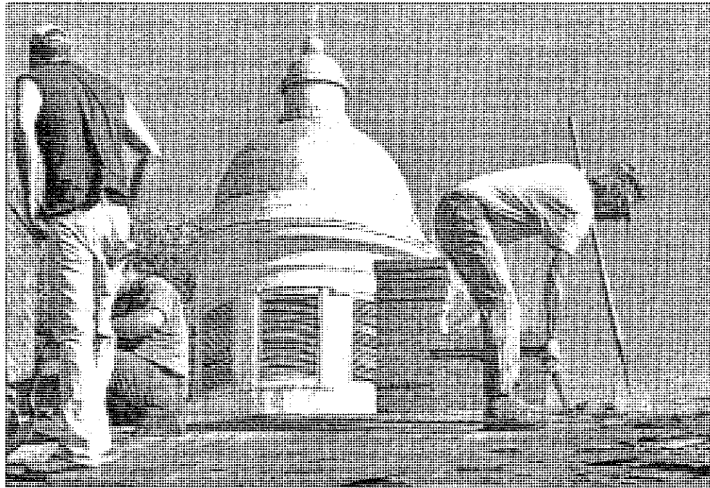
With the support of the Seneca County courthouse as the background, volunteers met to work on Ovid on Saturday, Aug. 27. They are repairing the roof on the former surrogate clerk's office, one of the three buildings making up the courthouse complex in the village. Two of the three buildings were found to need a new roof. The courthouse roof is to be replaced at a later date.
